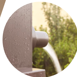
Controlled rainwater drain
